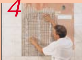
Press the mirror heating mat into the tile adhesive – make sure it is even and fixed. Then cover the mat with tile adhesive – make sure the surface is smooth.
